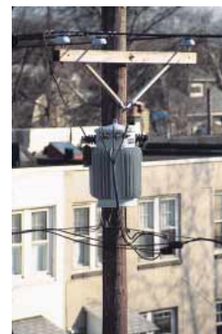
This cylindrical step-down transformer drops the voltage from 4 000 V to 220 V for delivery to a group of residences. (George Semple)
