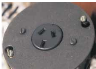
Figure 28.29 A power connection for a 240-V appliance.
