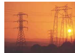
Figure 27.15 Power companies transfer electrical energy at high potential differences.
