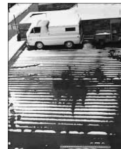
Melted snow pattern on a parking lot surface indicates the presence of underground hot water pipes used to aid snow removal. Energy from the water is conducted from the pipes to the pavement, where it causes the snow to melt.
